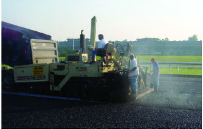
Crews from ATS Construction paving the porous drainage layer for the track.
