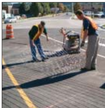
Workers lay steel grids on reheated asphalt to create the brick imprint.
