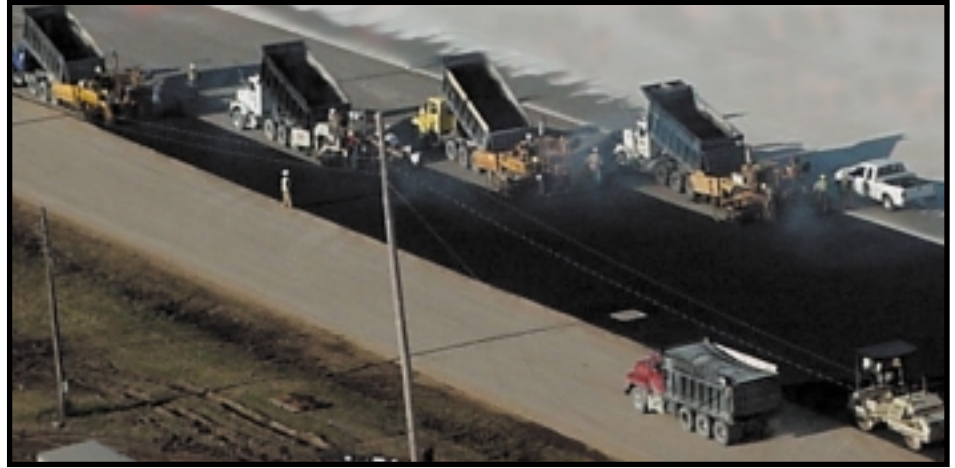
Rogers Group paving part of the runway at Ft. Campbell Keyhole Hardstand Area
