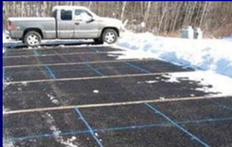
Figure 5. Porous asphalt parking lot one hour after being plowed. Photo courtesy of the University of New Hampshire Stormwater Center
